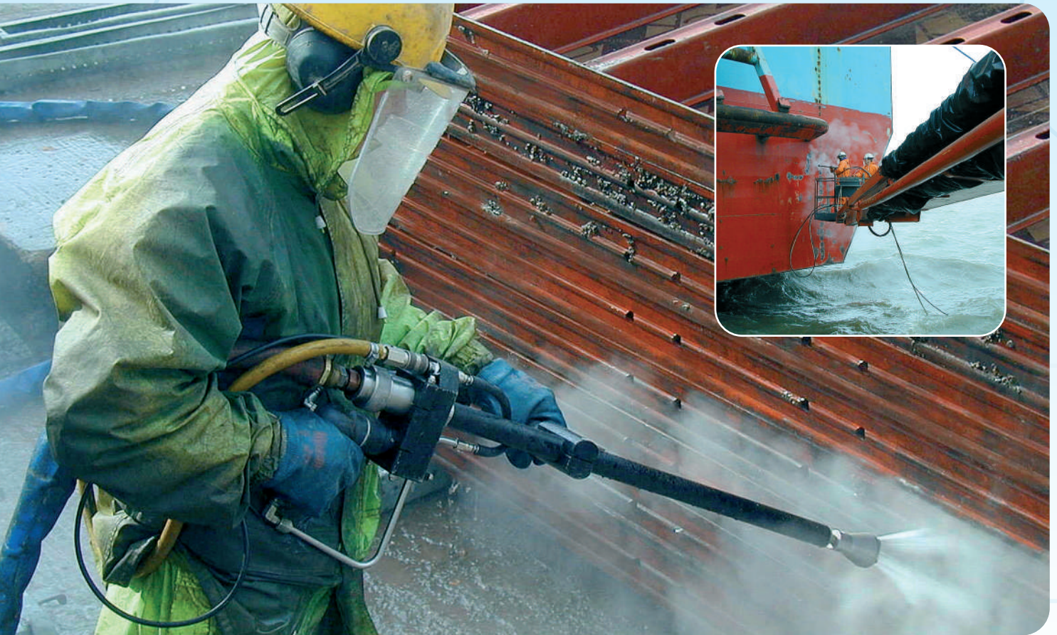
Main Picture: Stripping concrete from formwork at 2500 bar Inset: Surface preparation, shiprepair at 3000 bar
